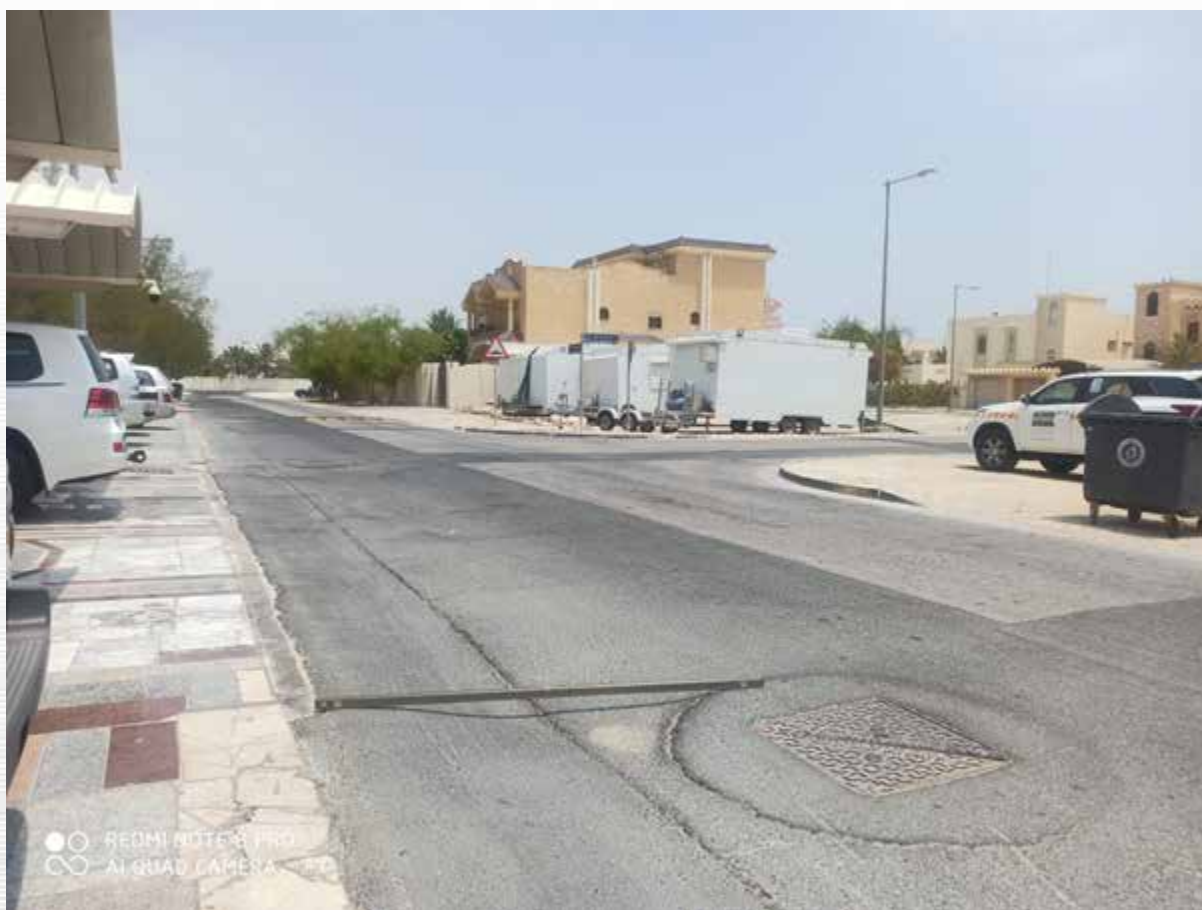
Figure 7-6 Depressions around manhole covers – Umm Al-Hawaya St
